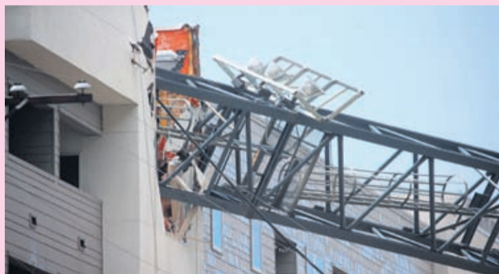
In this June 9, 2019, file photo, officials respond to the scene after a crane collapsed into Elan City Lights apartments amid severe thunderstorms in Dallas.
